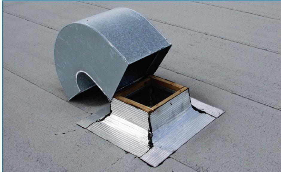
Figure 4-85: This gooseneck was attached with only two small screws. A substantial amount of water was able to enter the building during Hurricane Francis. (Florida, 2004)
