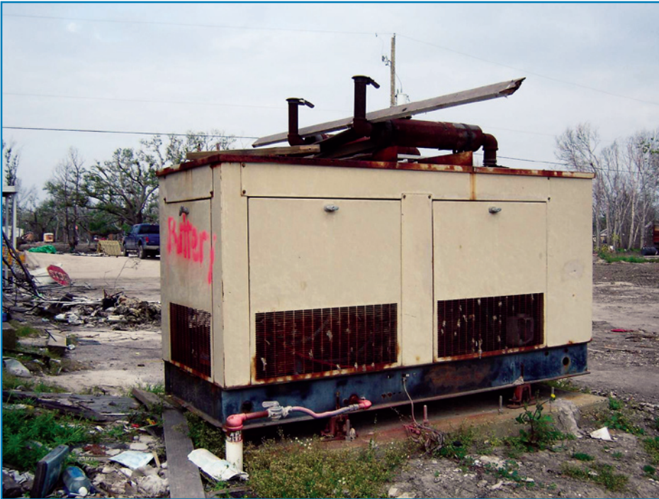
Figure 3-21: Although it was anchored and not displaced by floodwaters, this generator was out of service after being submerged (Hurricane Katrina, 2005).
