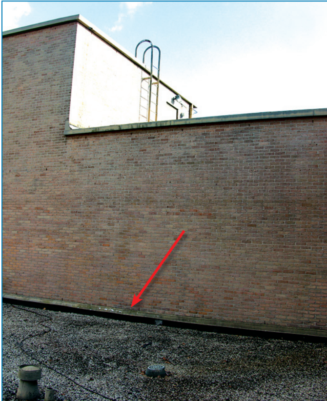
Figure 4-58: Water leaked inside along the base of the brick veneer walls (red arrow). Hurricane Katrina (Louisiana, 2005)
