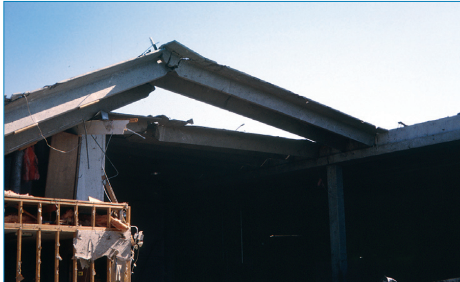
Figure 4-32: Twin-Tee roof panel lifted as a result of the combined effects of wind uplift and pre-tension. Tornado (Missouri, May 2003)
