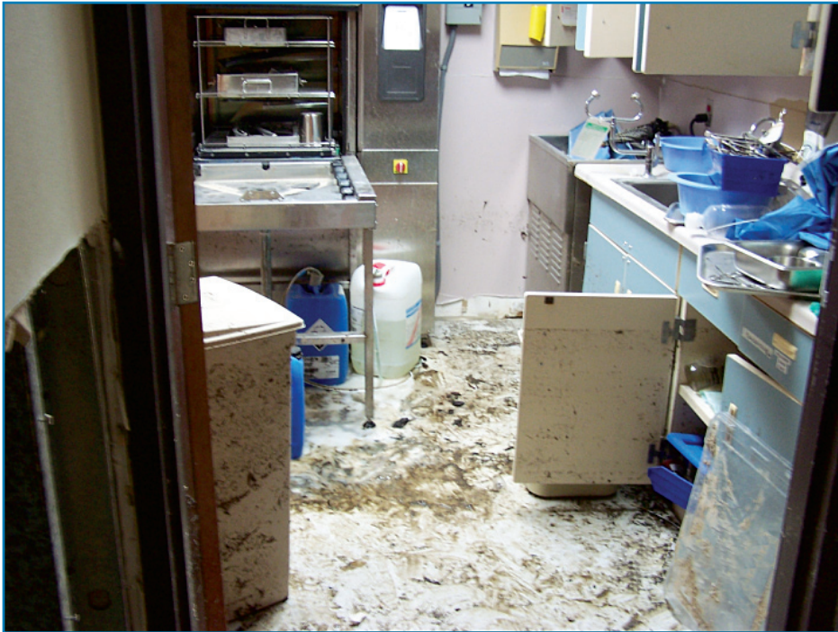
Figure 3-23: The interior of the Hancock Medical Center required extensive cleanup following flooding (Hurricane Katrina, 2005).
