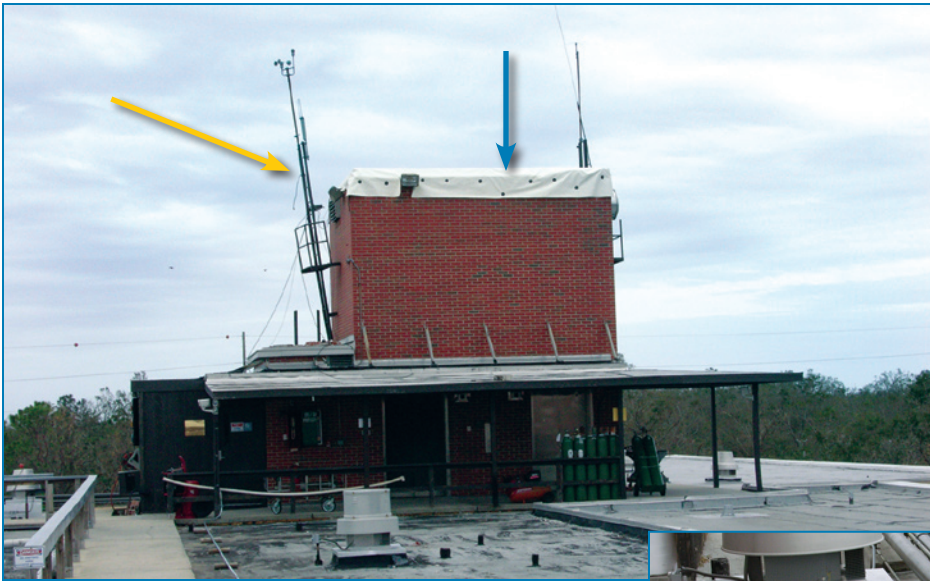
Figure 4-126: The roof covering blew off – an emergency roof covering had been installed (blue arrow). The failure was caused by the inadequately attached nailer (see inset). The leaning mast at the right is a ladder (yellow arrow), with an extension for communications and an anemometer for the nearby heliport.
