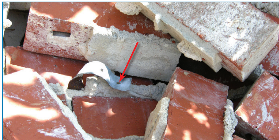
Figure 4-53: This tie remained embedded in the mortar joint while the smooth-shank nail pulled from the stud.
