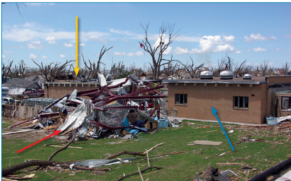
Figure 4-131: The building housing the generator is shown by the yellow arrow. The kitchen facility is shown by the blue arrow. The red arrow shows the collapsed storage building.
