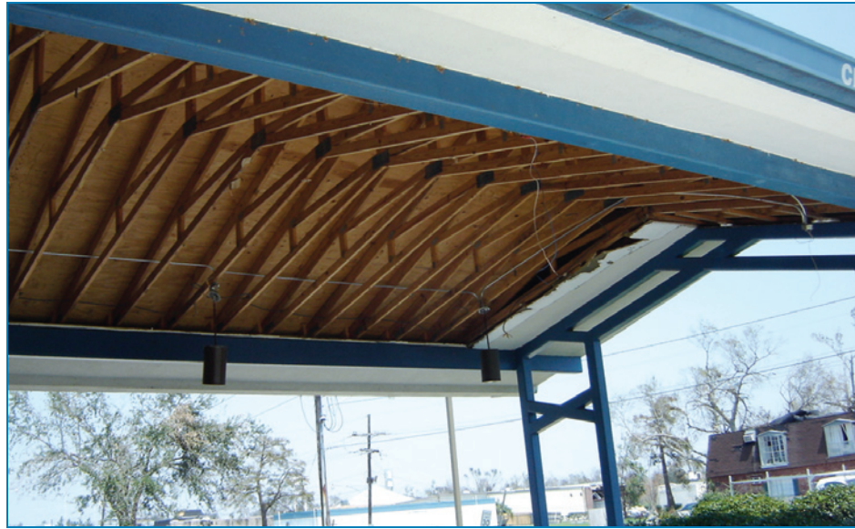
Figure 4-50: Hospital canopy damage. Hurricane Katrina (Louisiana, 2005)
