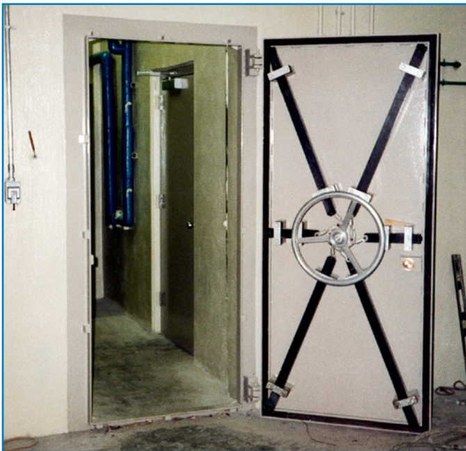
Figure 3-36: Permanent watertight doors designed for deep water
