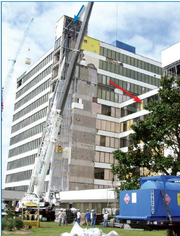
Figure 4-18: Broken windows in the connecting walkway between the hospital (right) and MOB (left) (red arrow). Also note the broken windows and loss of EIFS (including the gypsum board on both sides of the studs) at the elevator enclosure (blue arrow).
