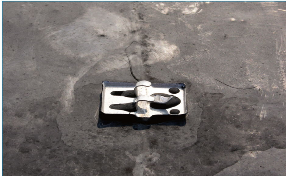
Figure 4-100: The conductor deformed the prongs under wind pressure, and pulled away from the connector. Hurricane Katrina (Mississippi, 2005)
