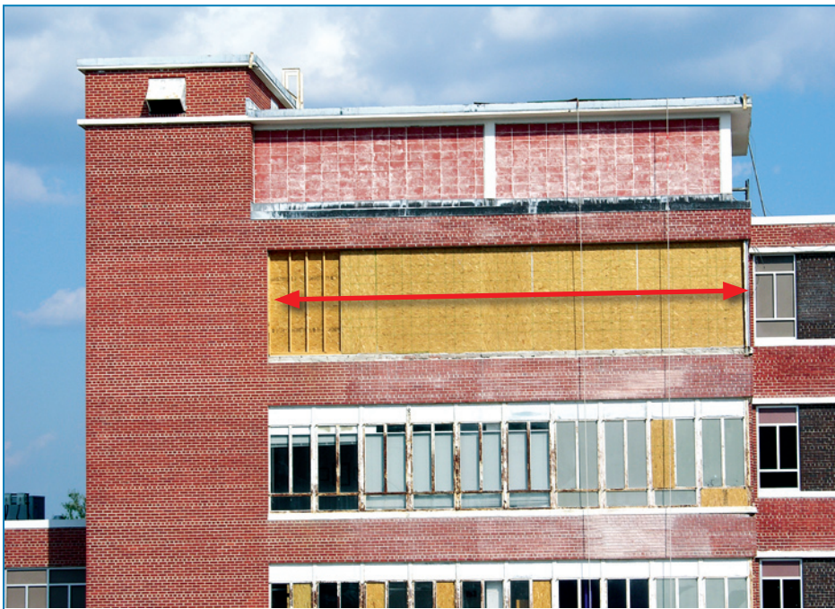
Figure 4-115: Wind pressure caused the window frames on the upper floor to fail (red arrow). Hurricane Katrina (Mississippi, 2005)
