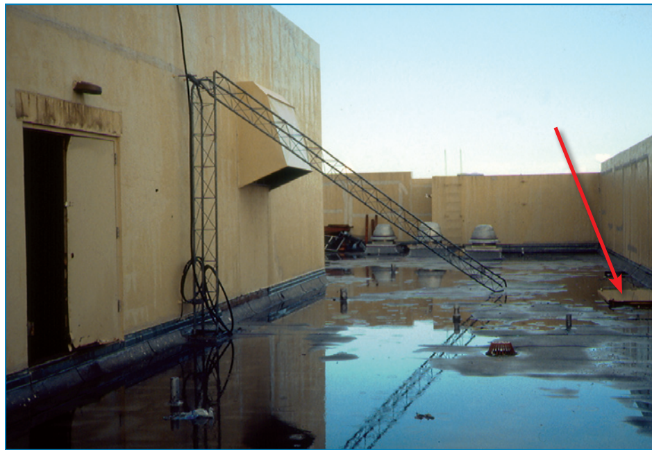
Figure 4-121: The antenna at this hospital collapsed and was whipped back and forth across the roof membrane. Hurricane Andrew (Florida, 1992)
