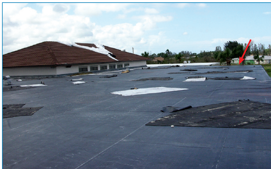
Figure 4-69: The original modified bitumen membrane was blown away after the gutter lifted in the area shown by the red arrow (the black membrane is a temporary roof). Hurricane Francis (Florida, 2004)
