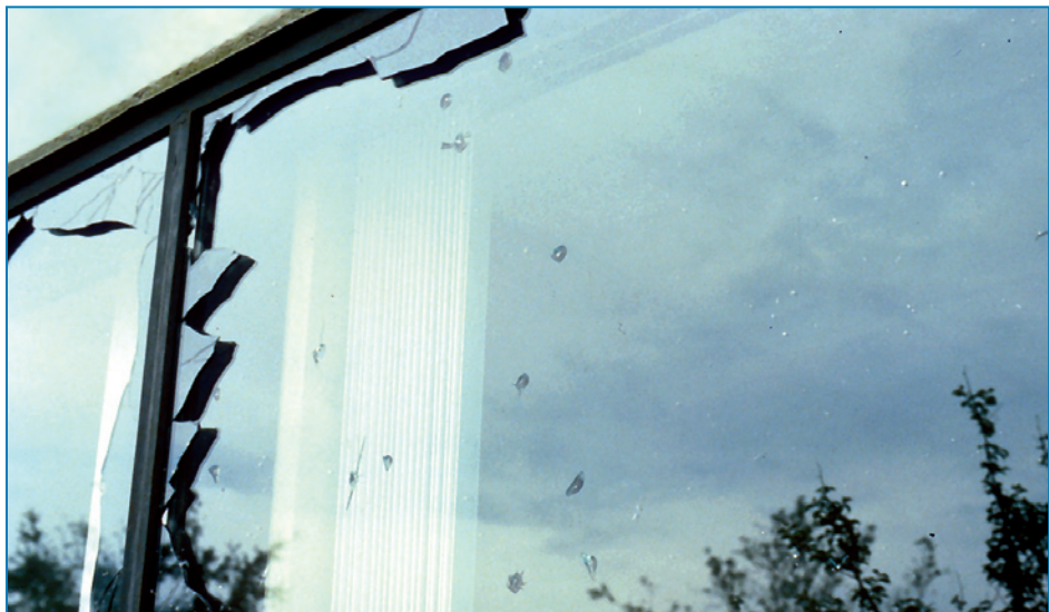
Figure 4-10: The outer window panes were broken by aggregate from a built-up roof. Hurricane Hugo (South Carolina, 1989)
