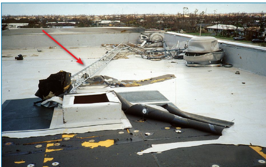
Figure 4-95: The collapse of the antenna tower caused progressive peeling of the roof membrane. Also note that the exhaust fan blew off the curb, but the high parapet kept it from blowing off the roof. Hurricane Andrew (Florida, 1992)
