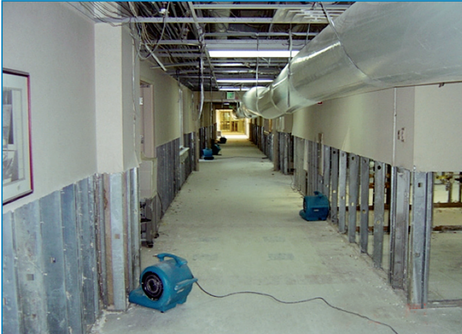
Figure 3-18: Drying out the ground floor at Hancock Medical Center (Hurricane Katrina, 2005)
