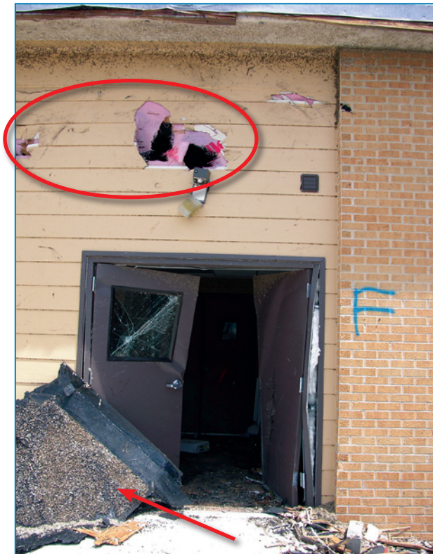
Figure 4-134: The BUR missile (red arrow) struck the right door. Missiles also punctured the siding and wood sheathing (red oval).
