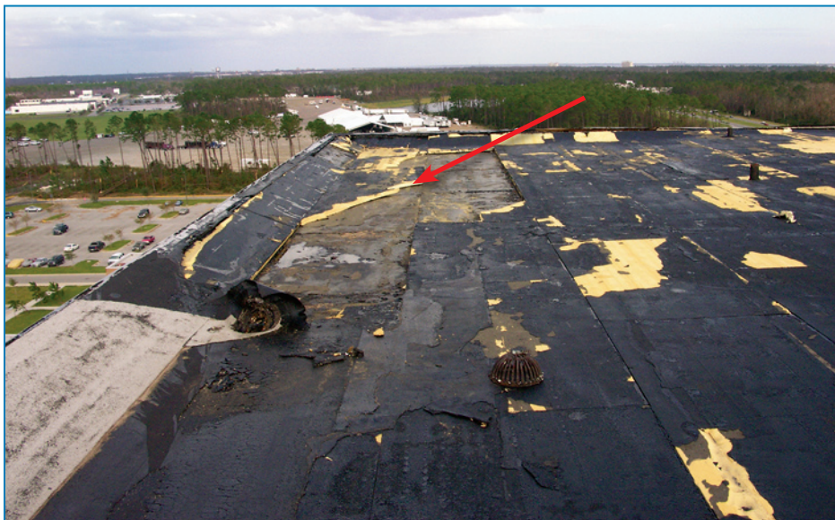
Figure 4-71: The blown off insulation (red arrow) may have initiated blow off of the roof membrane. Hurricane Ivan (Florida, 2004)
