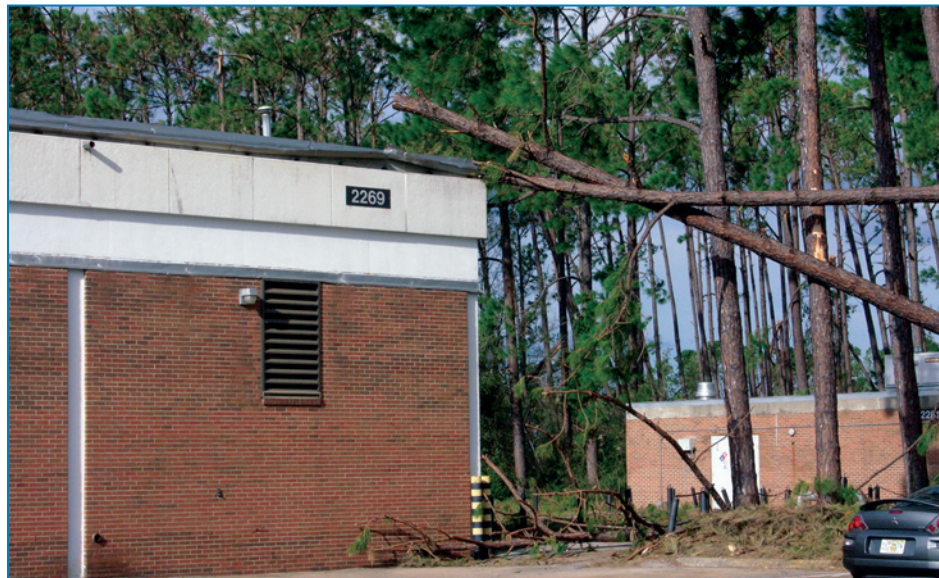
Figure 4-24: The roof membrane on this hospital's materials management facility was ruptured by falling trees. Hurricane Ivan (Florida, 2004)
