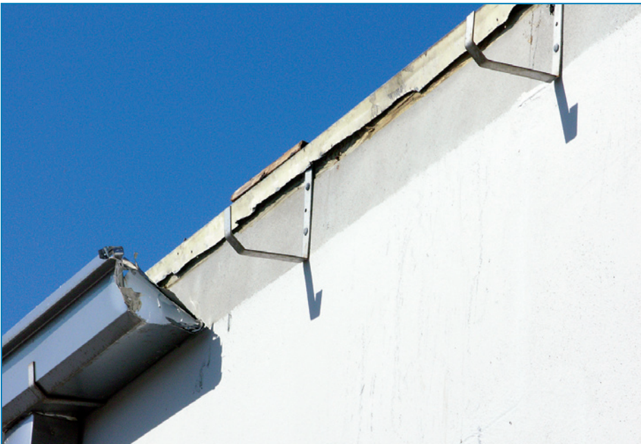
Figure 4-68: This gutter, supported by a type of bracket that provides no significant uplift resistance, failed when wind lifted it, together with the metal edge flashing that lapped into the gutter. Hurricane Francis (Florida, 2004)
