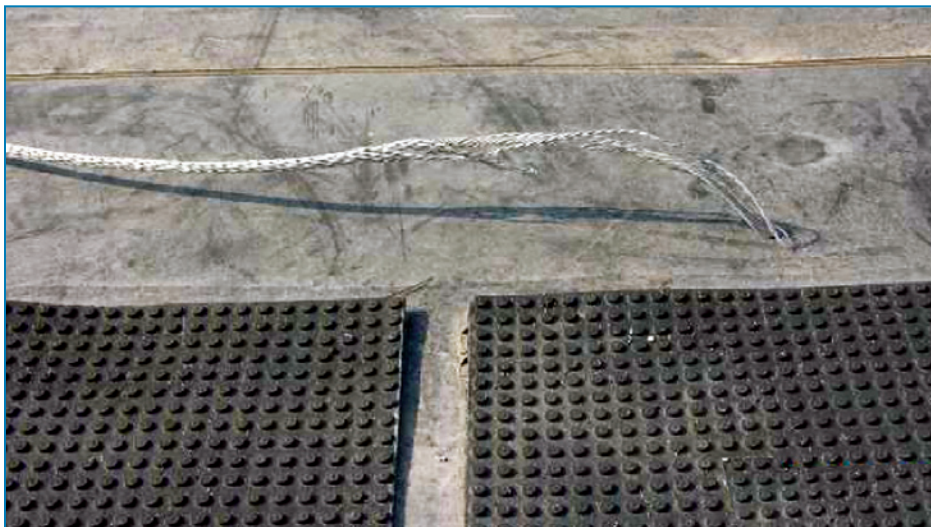
Figure 4-99: View of an end of a conductor at a hospital that became disconnected. Hurricane Katrina (Mississippi, 2005)
