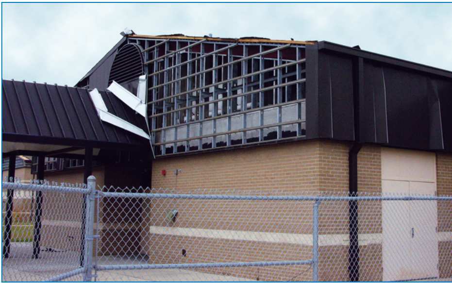
Figure 4-62: The loss of metal wall panels allowed a substantial amount of wind-driven rain to penetrate this building. Hurricane Ivan (Florida, 2004)
