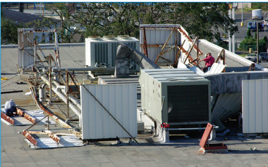
Figure 4-94: Equipment screen panels, such as these blown away at a hospital, can break glazing, puncture roof membranes, and cause injury. Hurricane Ivan (Florida, 2004)
