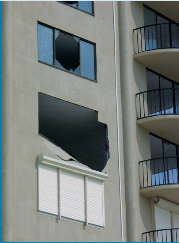
Figure 4-118: The lower window assembly was protected with a motorized shutter. Hurricane Ivan (Florida, 2004)
