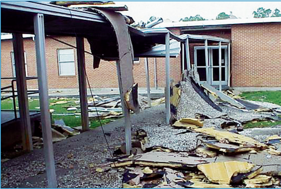
Figure 4-27: Open walkways do not provide protection from wind-borne debris. (Hurricane Katrina, Mississippi)
