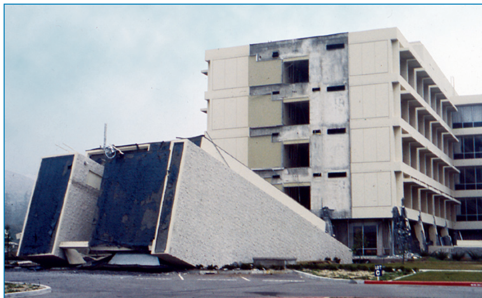
Figure 2-21: Collapsed stair tower in main building of Olive View Hospital
