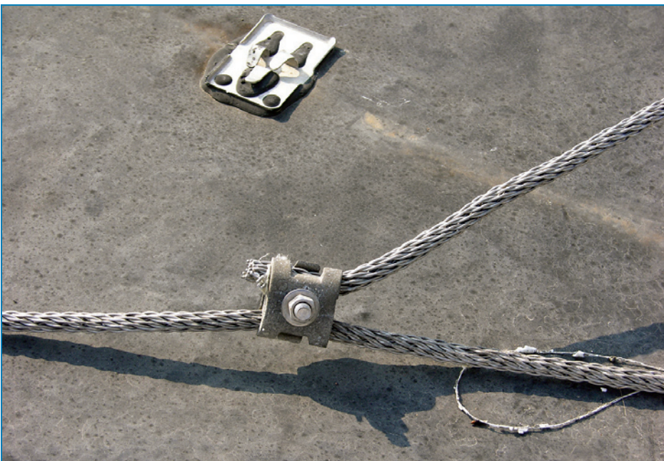
Figure 4-105: Bolted splice connectors are recommended to prevent free ends of connectors from being whipped around by wind. Hurricane Katrina (Mississippi, 2005)
