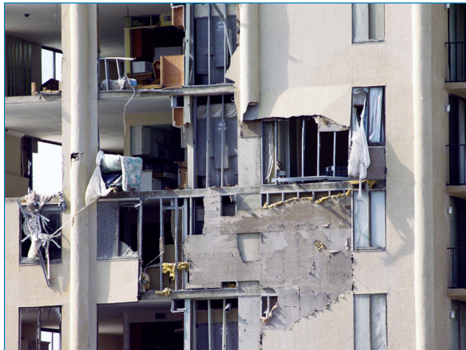
Figure 4-61: The stucco wall failure was caused by inadequate attachment between the stud tracks and the building's structure. Hurricane Ivan (Florida, 2004)
