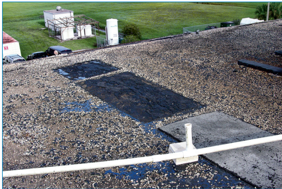
Figure 4-82: View of the back side of the third floor roof where the gutter and an asphalt plank walkway pad were blown away. The loose aggregate surfacing was also blown away.
