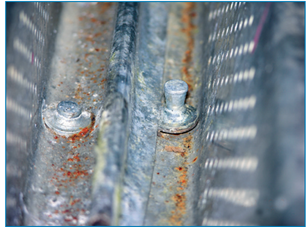
Figure 4-30: View looking along a sidelap of a deck attached with powder-driven pins. The right pin does not provide adequate uplift and shear resistance.
