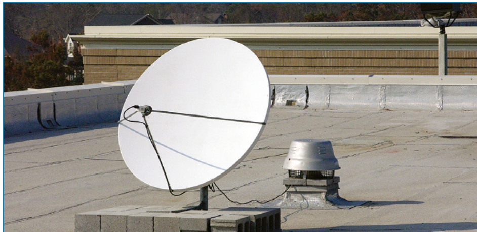
Figure 4-96: Common anchoring method for satellite dish. Hurricane Ivan (Florida, 2004)
