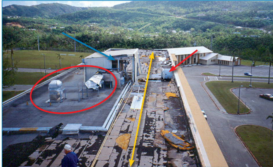
Figure 4-9: Damaged roof membrane and rooftop equipment. Typhoon Paka (1997)
