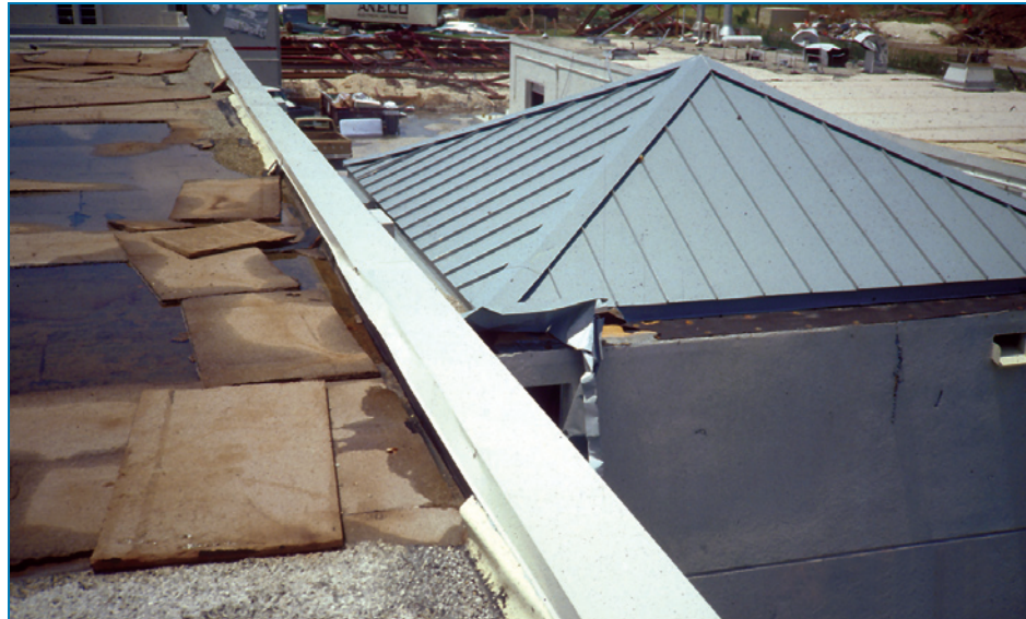
Figure 4-6: The irregularity created by the stair tower (covered with a metal roof) caused turbulence resulting in wind speed-up and roof damage. Hurricane Andrew (Florida, 1992)
