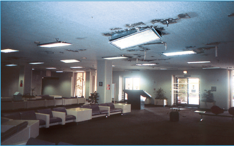
Figure 2-33: Damage to ceiling and fixtures from sprinkler breaks
