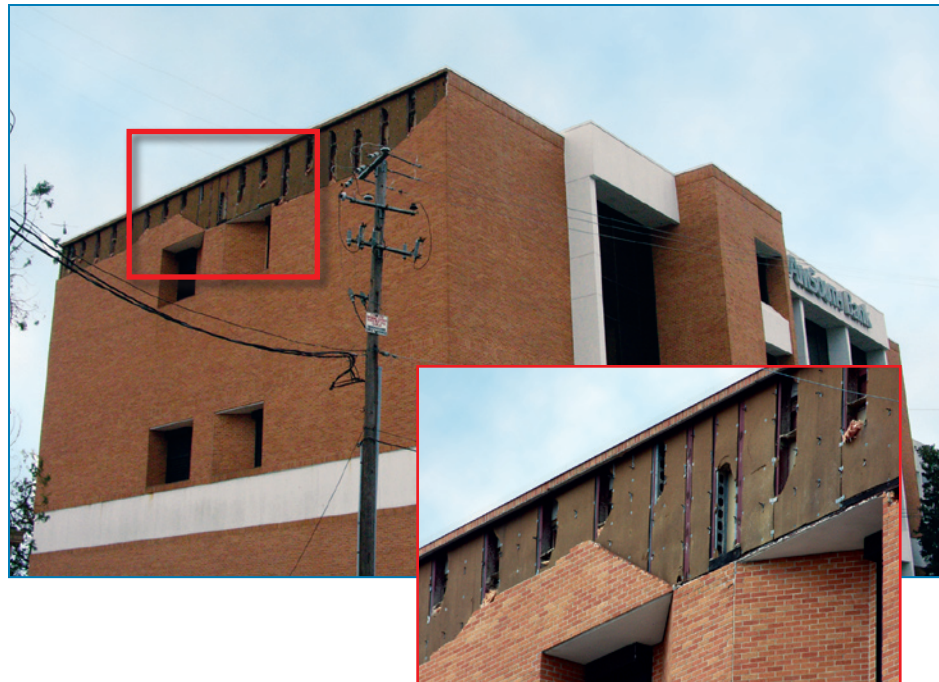
Figure 4-52: The brick veneer failure on this building was attributed to tie corrosion. Hurricane Ivan (Florida, 2004)
