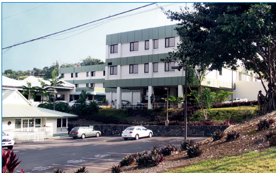
Figure 2-35: Kona Community Hospital. Addition (1989) supported on isolated columns in the foreground. The original building (1972) is in the left background.
