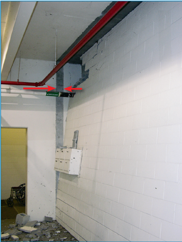
Figure 4-51: The red arrows show the original location of a CMU wall that nearly collapsed following a rolling door failure. Hurricane Charley (Florida, 2004)
