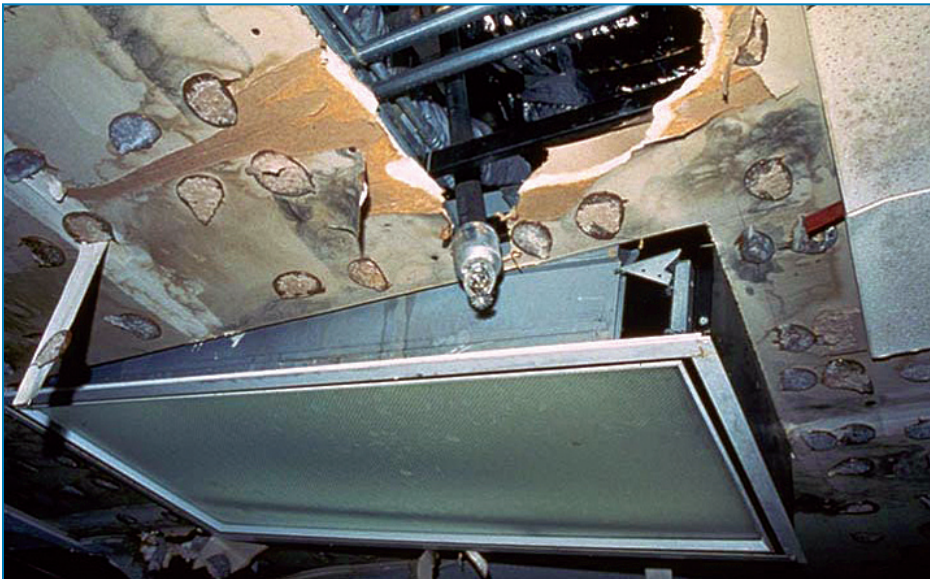
Figure 2-34: Detail of water damage to ceiling
