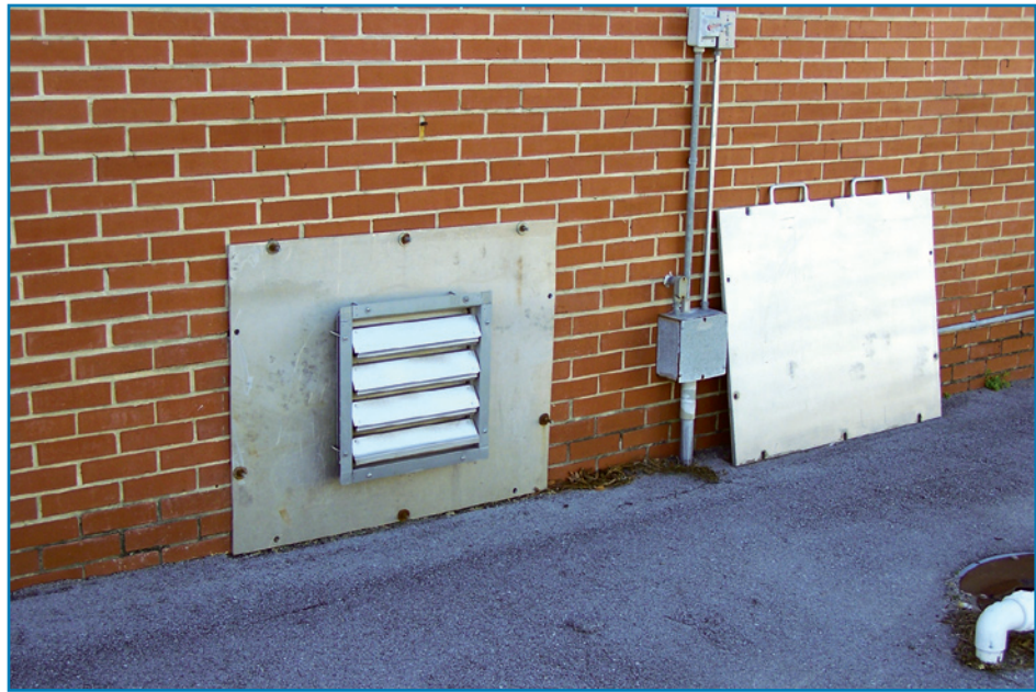
Figure 3-44: The ventilation openings for the original building's crawlspace are protected with floodproofing panels that are bolted in place when flooding is predicted.
