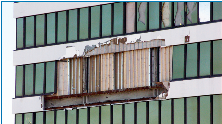
Figure 4-17: Broken windows in the MOB. Wood studs and gypsum board had been temporarily installed after the hurricane to prevent patients from inadvertently falling out of the MOB.
