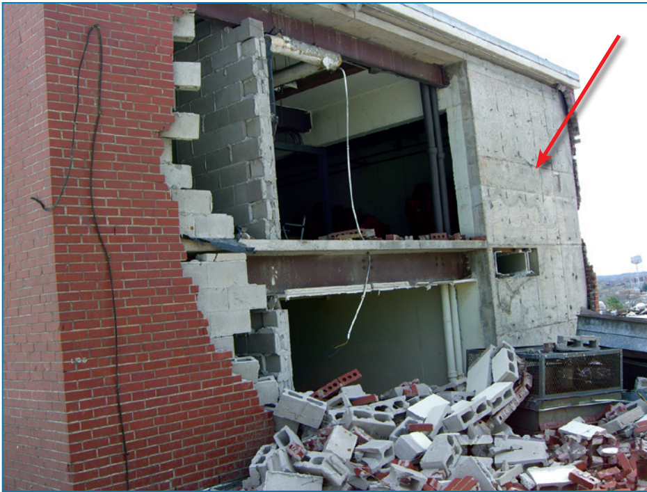
Figure 4-148: Collapsed brick veneer/CMU wall at a mechanical room. The cast-in-place concrete wall (arrow) remained, but the brick veneer was blown away.
