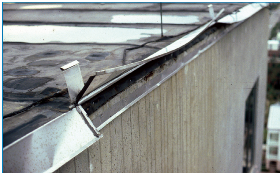
Figure 4-66: The metal edge flashing on this hospital disengaged from the continuous cleat and the vertical flange lifted. Hurricane Hugo (South Carolina, 1989)
