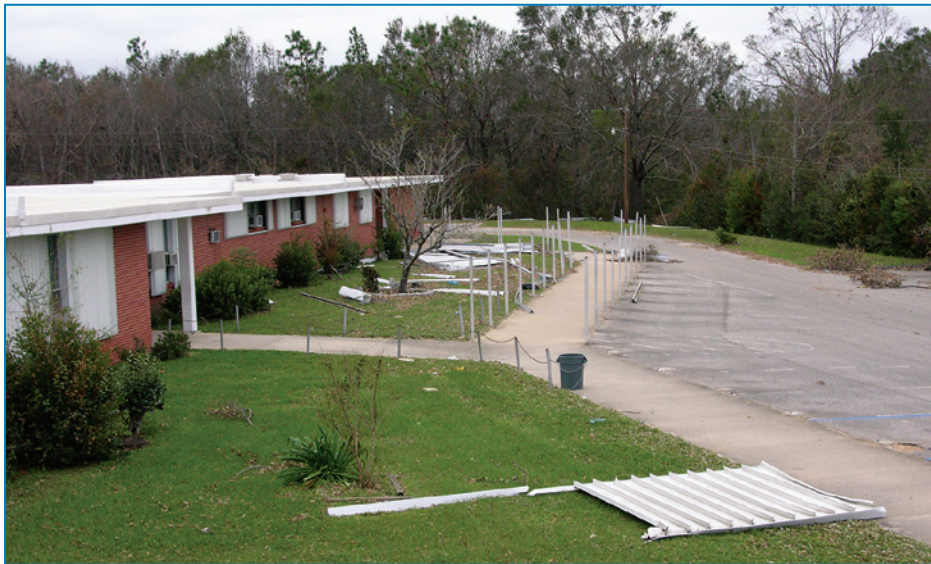
Figure 4-33: The destroyed walkway canopy in front of this building became wind-borne debris. Hurricane Ivan (Florida, 2004)
