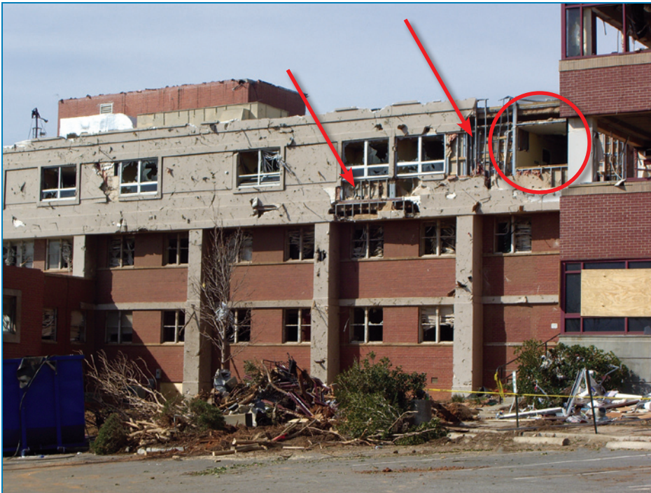
Figure 4-145: One window frame was blown away (red circle). The EIFS was penetrated by many missiles, and in some areas, the entire wall (except the studs) was blown away (arrows).
