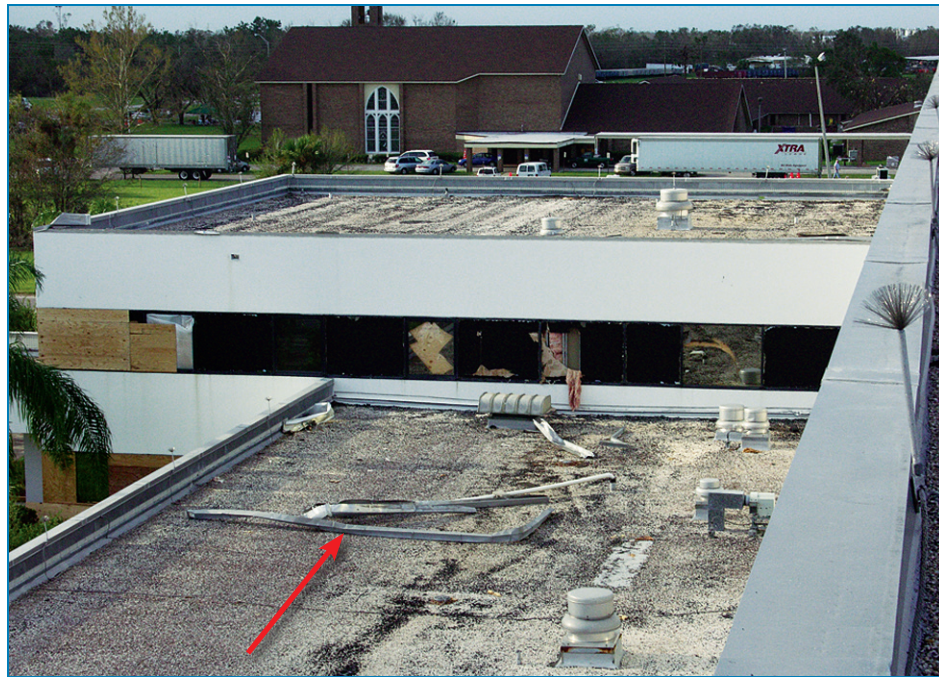
Figure 4-81: A view of the ICU from the third floor roof. The gutters (red arrow) are from the back side of the third floor roof.
